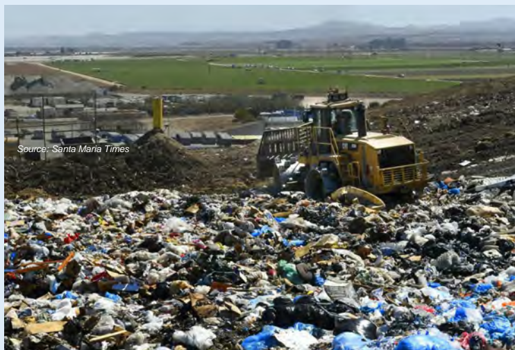
Collecting emissions from landfills is a complicated process, regulated at all local, State, and federal levels of government
