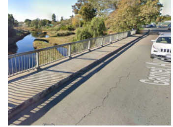
Figure 6. Narrow sidewalk on Rose Creek bridge
