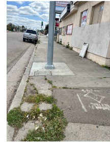
Figure 4. Unkept sidewalk between Woodman St. and 65th St.
