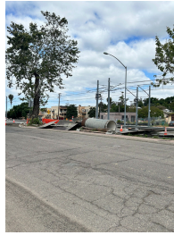
Figure 3. Safety hazard from construction material on the median at the intersection of 65th St. & Imperial Ave.
