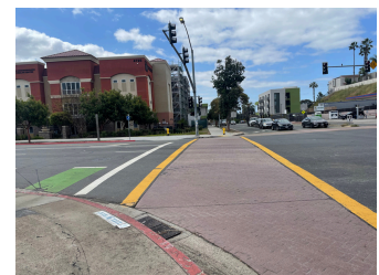
Figure 2. Curb not cut on Market St. and 47th St.
