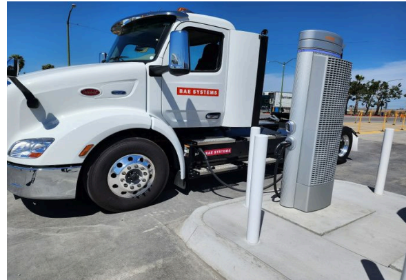
Figure 5. A DC fast charger installed by SDG&E at Truck Net, north of the Otay Mesa Port of Entry in California. Photo: SDG&E
